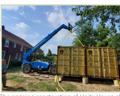
The ongoing construction of Unity House also prioritizes growing Detroit's work force. We partnered with and employed training orgs for welding and electrical work .
